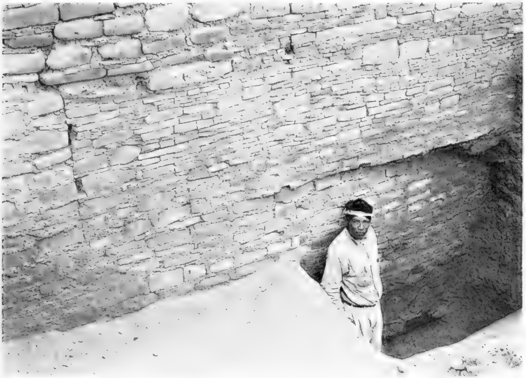
FIG. 163.—The overhang above the Indian's head shows the union of a new addition with older, partially razed walls in Pueblo Bonito. (Photograph by Neil M. Judd. Courtesy of the National Geographic Society.)
